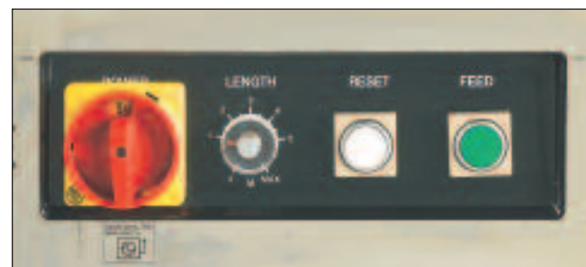
OPERATOR FRIENDLY CONTROL PANEL
